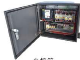
电控箱 Electric control box
